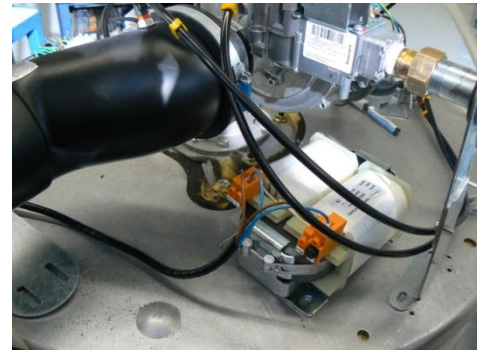
Fig. 1 - Position of transformer
